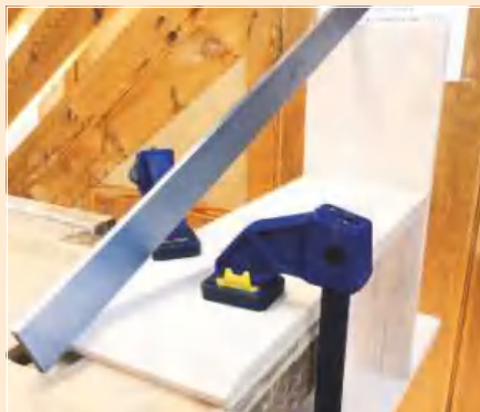
▲ Pic.27 Another way to check if the angles were correct was to line up every corner with the straightedge
